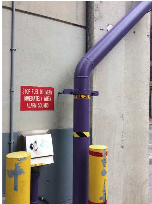
Photograph 11: Evidence of fuel diesel and/or fuel oil tanks at neighbouring 10 Shuter Street, to the east of the Site, facing southeast.
